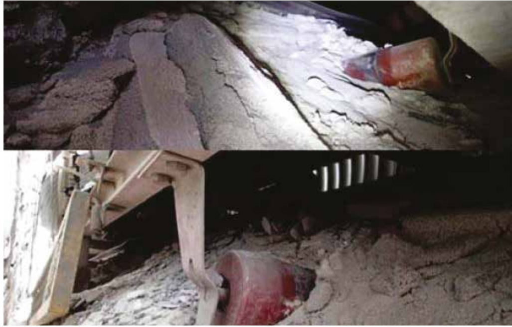
Boşaltım bölgesinde dökülen malzeme, ruloyu tamamen sarmış durumda. Telif Hakkı © Martin Engineering 2023 The roller is encapsulated by spillage at the discharge zone. Copyright © Martin Engineering 2023
